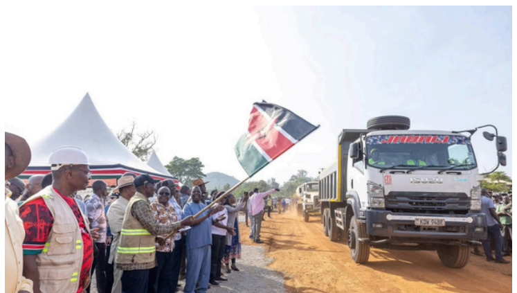
H.E. President William Ruto presided over the launch of the construction works for the 22 km Matayos–Nangina and Nangina–Sio Port–Mumbaka Roads in Busia County on 18th March 2026
