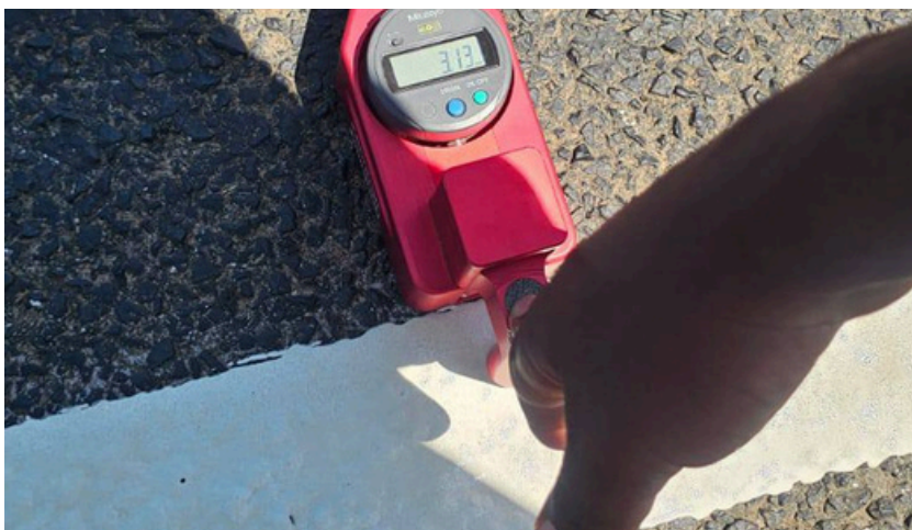
Road Marking Technology: Using a retroreflectometer to assess the retroreflectivity and thickness of thermoplastic road marking paint.
