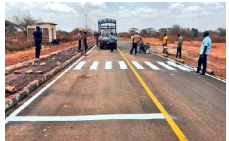
Mandera County: The 2 KM Banisa Town Roads project is now substantially complete, improving mobility, reducing dust, and enhancing access to markets, schools, and health facilities.
