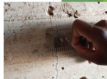
Crack width measurement using a scale
