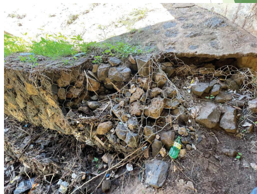
Dilapidated gabion mesh.
