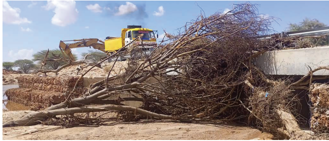
Photo showing driftwood blocking a box culvert
