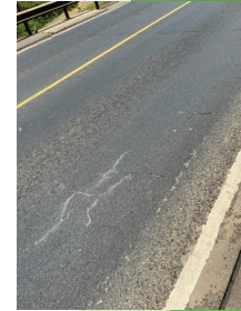
Crack on pavement.
