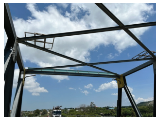
Vandalization of the lighting facility.
