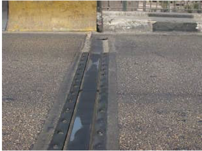
Rubber faceplate type: -Worn-out/ damaged surface rubber.
