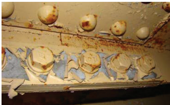
Deterioration of corrosion protection
