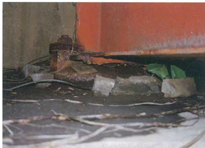
➤ Broken mortar seat.
