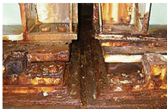
Corrosion of bearings.
