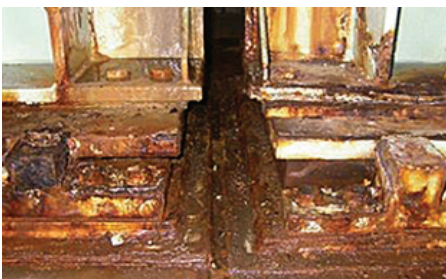
Girder ends with frequent water leakage
