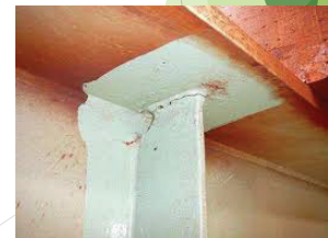
Cracks on steel member.
