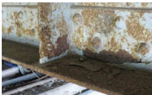
Corrosion of bottom flange
