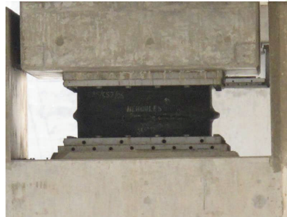
Rubber bearing (damaged).
