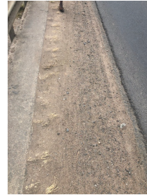
Clogging of the drainage facilities.
